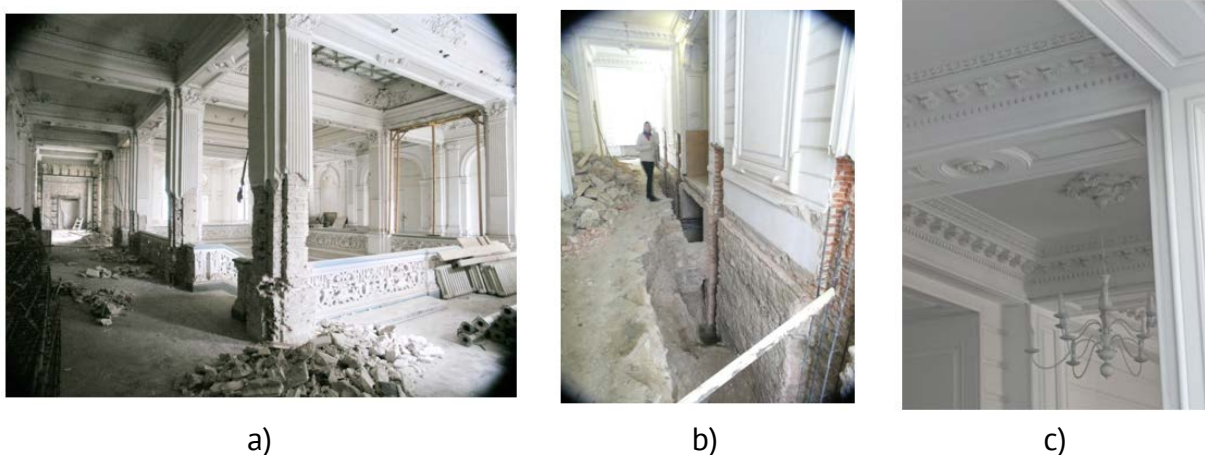
Figure 5. (a, b) Restoration works in the National Museum of Plastic Arts of Moldova; (c) Stylistic combinations in the ornamental decoration of the National Museum of Plastic Arts of Moldova.
