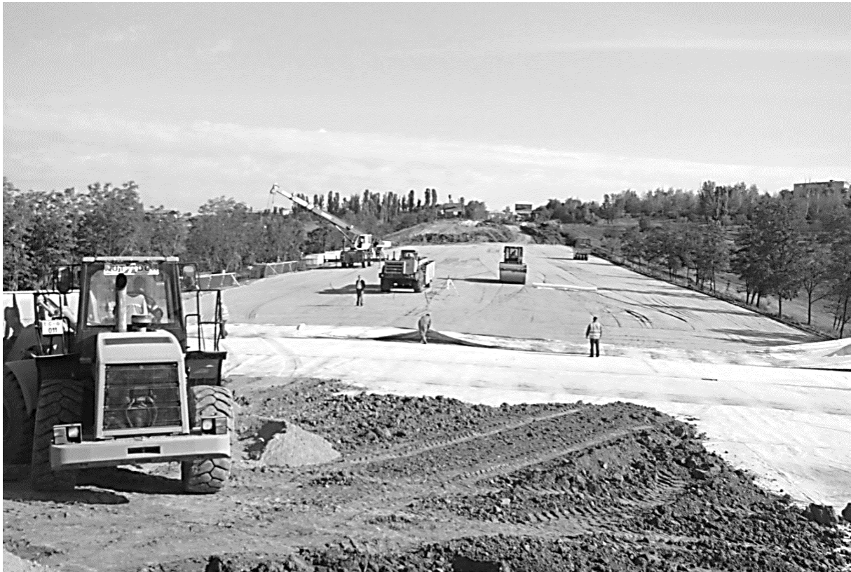
Figure 1. Restoration work at a site of embankment bypassing the town of Ialoveni.
