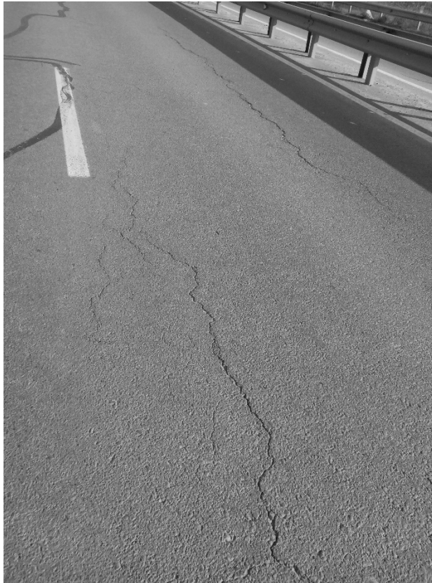
Figure 5. Longitudinal cracks in the road surface. December 2019.
