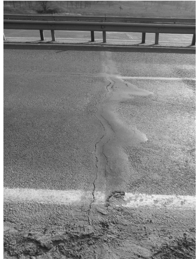
Figure 6. Transversal cracks in the road surface. December 2019.
